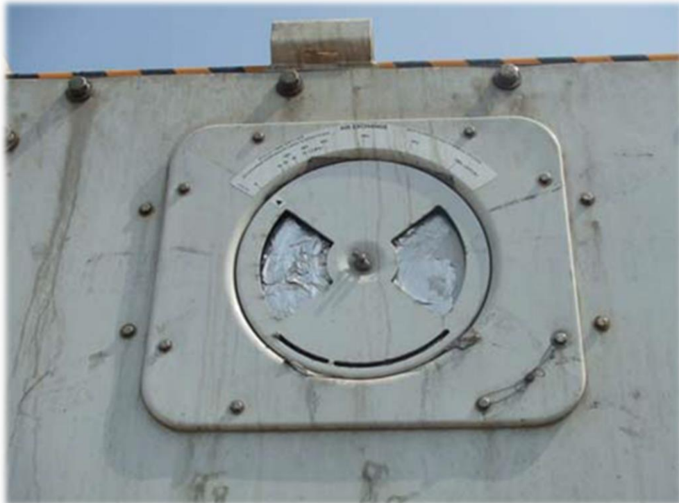
Air fresh cover incorrectly sealed with tape.
